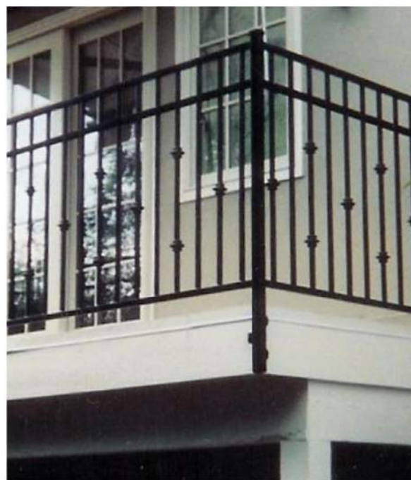
H METAL RAILING
